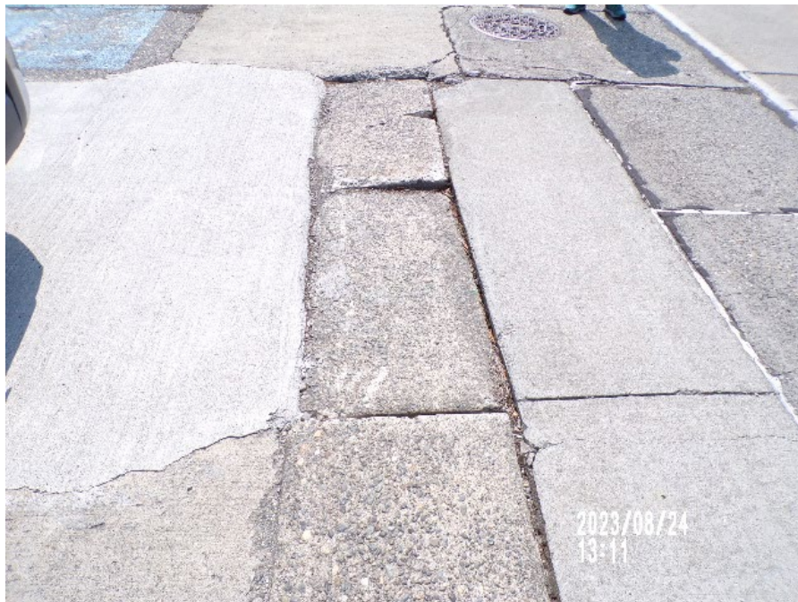
Photograph 8. August 2023 View facing south, cracked pavement in front of Building 15, OU2 Area 7.
