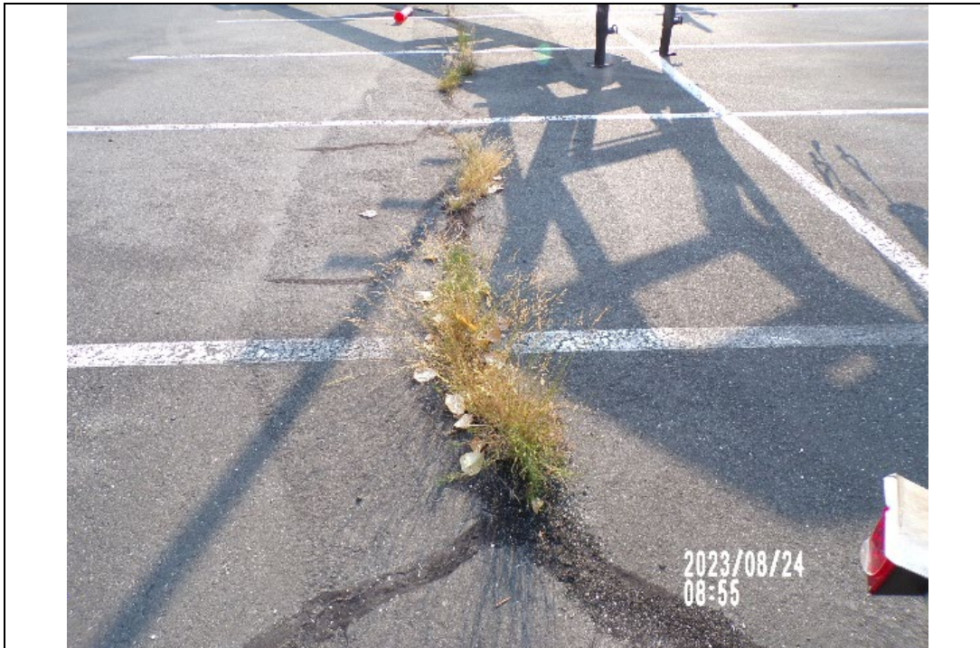
Photograph 1. August 2023 View of the site facing north pavement crack OU1 Area D.
