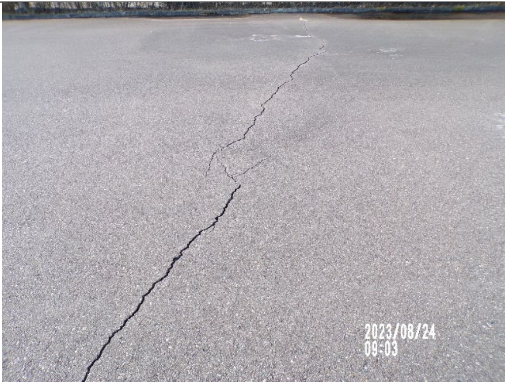
Photograph 4. August 2023 View facing south, pavement cracking near storage shed.
