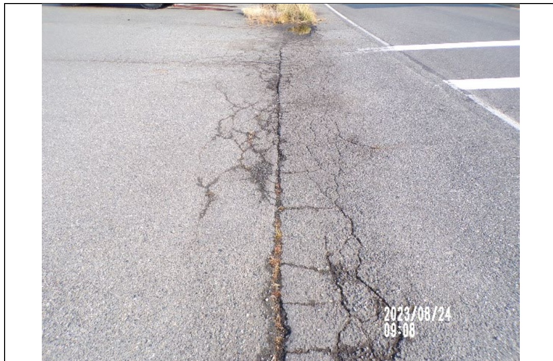
Photograph 2. August 2023 View facing north, alligating on east edge of OU1.
