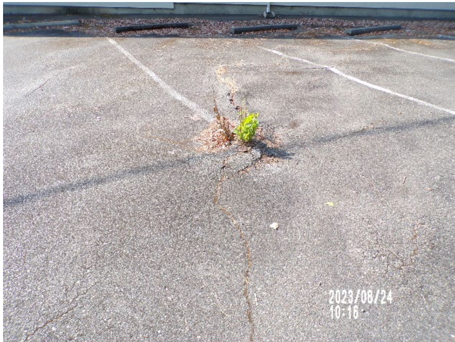
Photograph 7. August 2023 View facing south, root damage to asphalt at OU2 Area 2.
