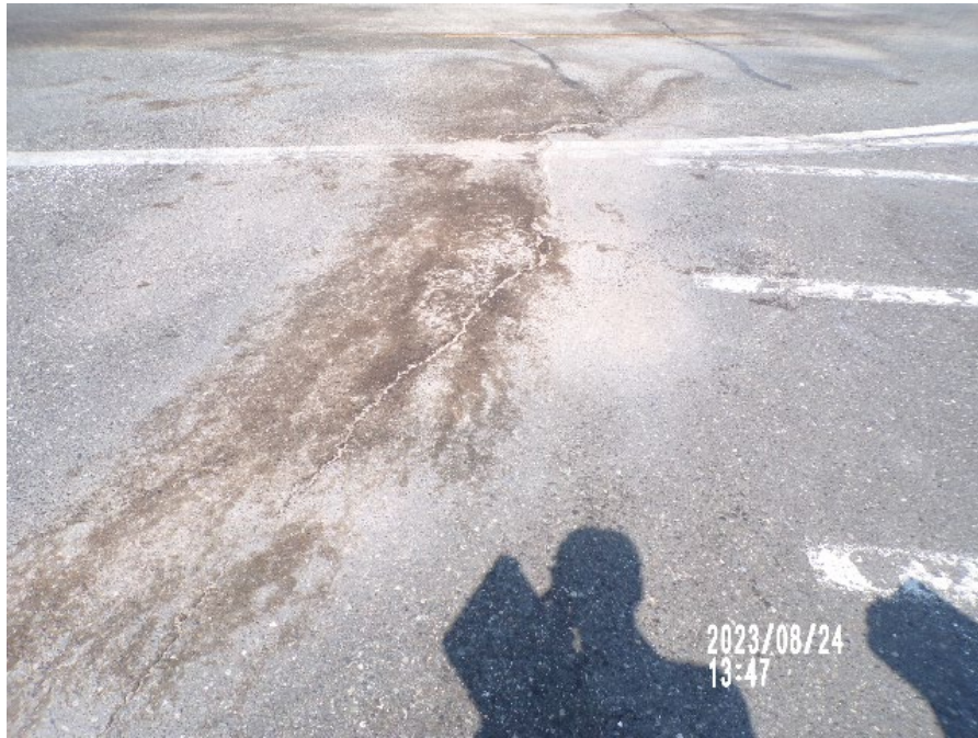
Photograph 10. View facing north, cracked pavement at OU2 Area 2. August 2023
