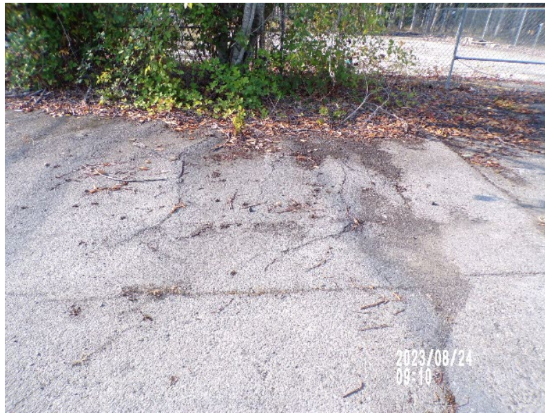
Photograph 5. View facing south, pavement cracking near southern plantation. August 2023
