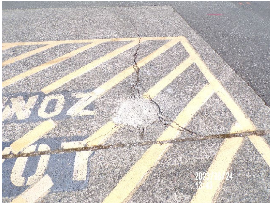
Photograph 9. View facing east, damaged pavement at loading zone OU2 Area 7. August 2023
